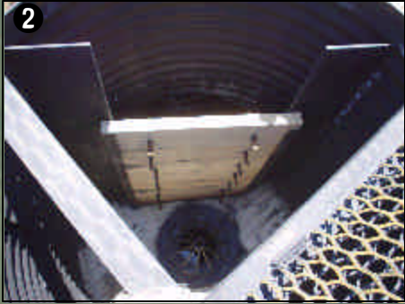
Stop Logs Inside Main Water Control Structure
